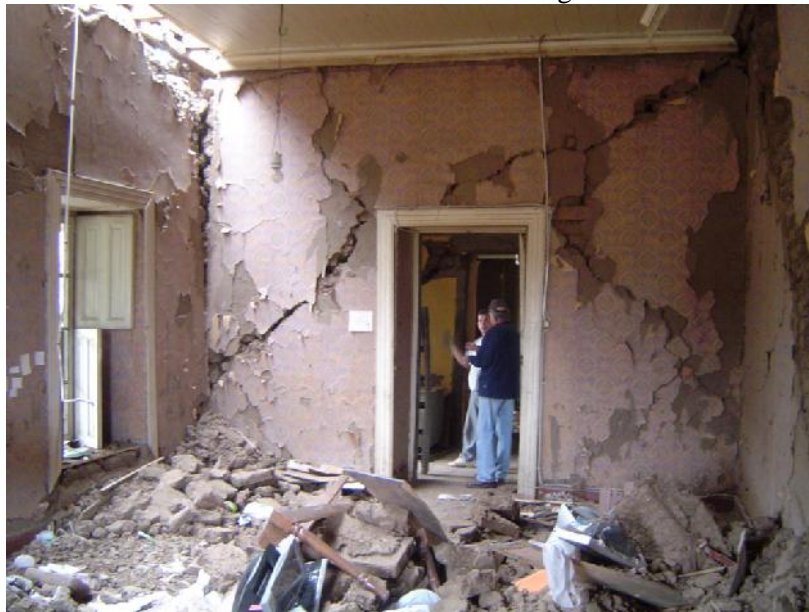
Figure 1: The use of adobe or earth-based brick masonry is quite extended in many seismic-prone countries; an integrated design has to consider this fact and evaluate it for promoting identity (Photo by the author)
