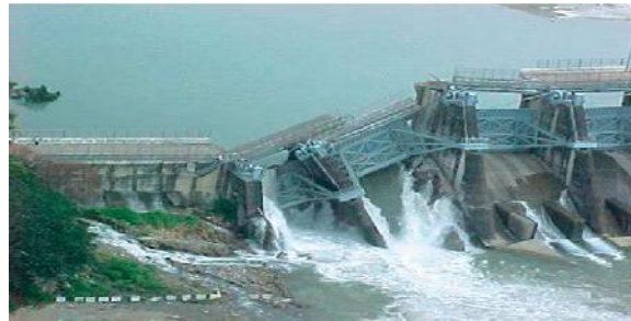
Figure 2: Break of the Shih Kang Dam
